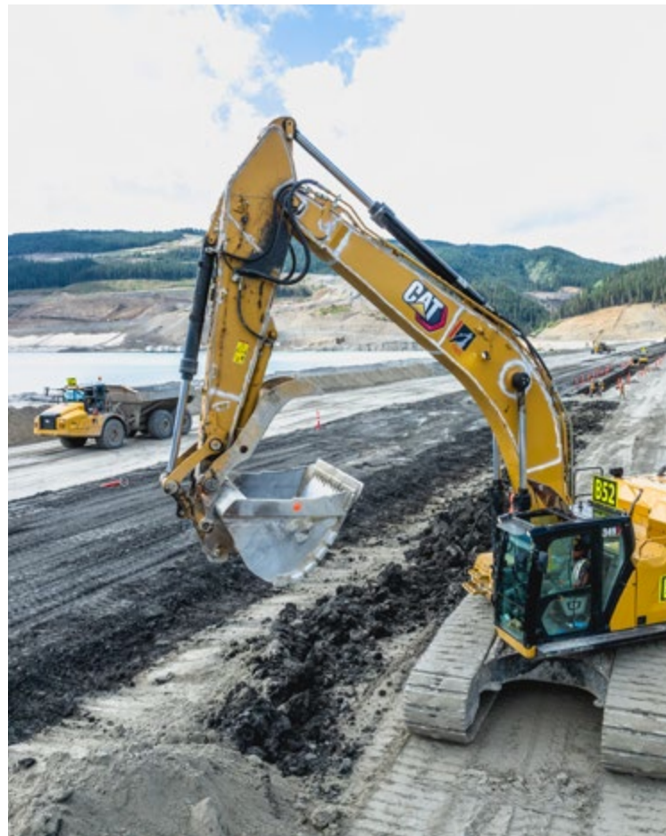
Above: TNDC equipment at work at the Red Chris mine TIA construction.
