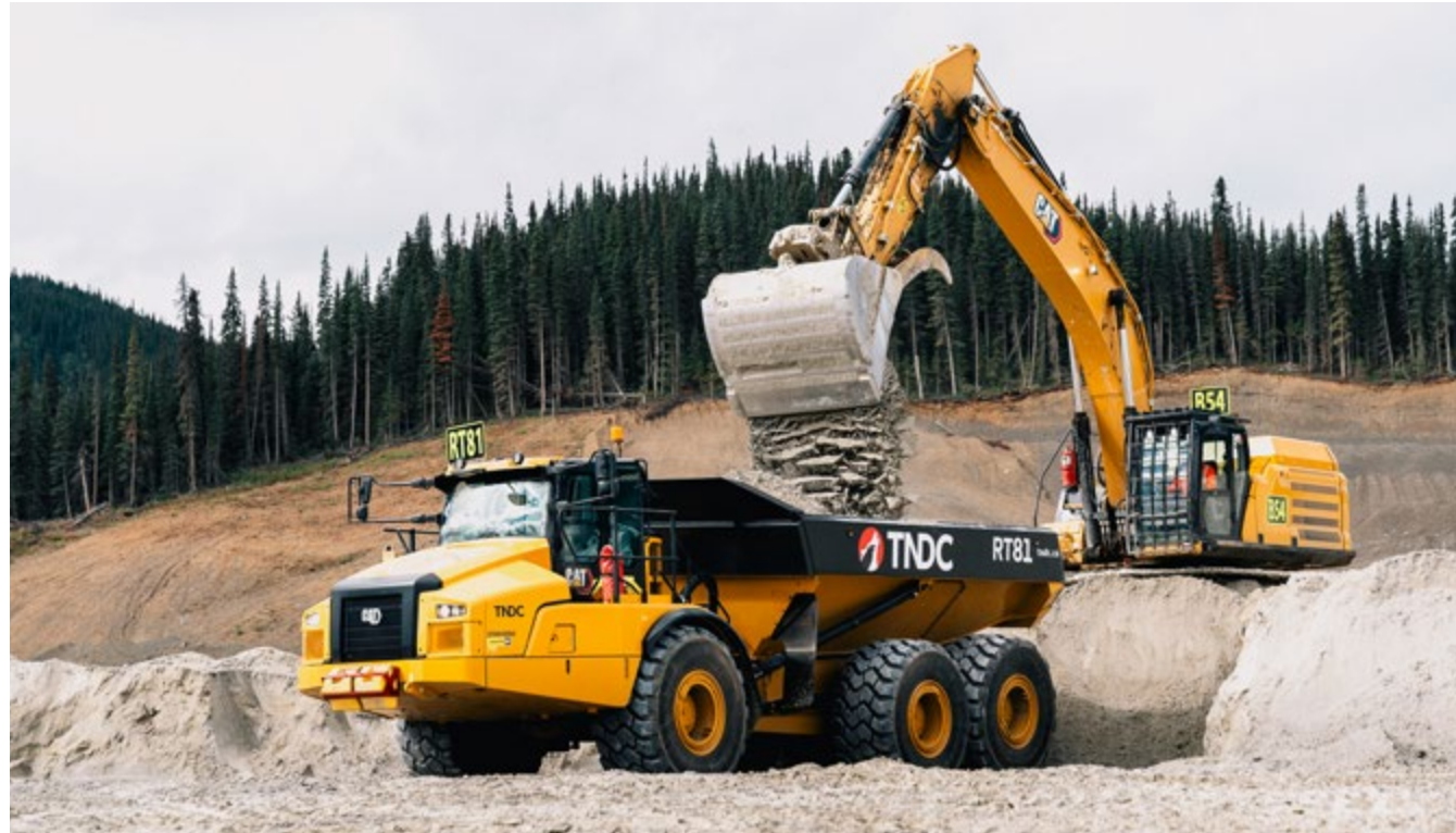
Above: TNDC equipment at work on our Red Chris TIA project site.
